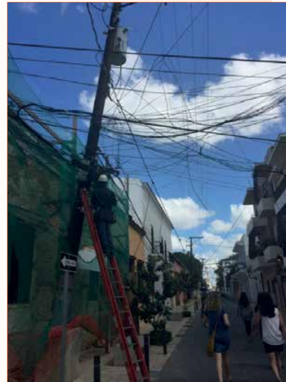
Figure 1: aerial power lines in Dominican Republic
