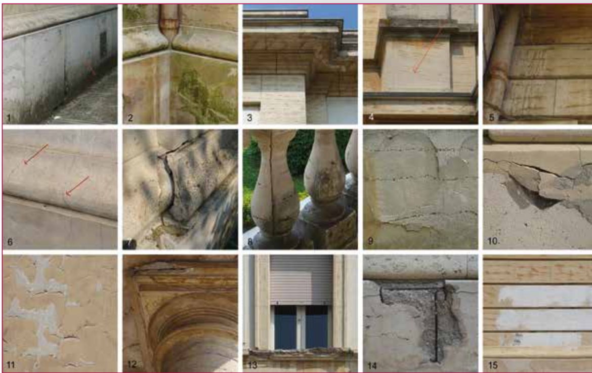
Fig. 9 - Summary of the degradation forms observed on the city hall facades: 1. superficial deposit; 2. biological coating; 3. scaling; 4. pulverisation; 5. run-off; 6. superficial cracking; 7-8. deep cracking; 9. swelling; 10. detachment; 11. paint layer detachment; 12. lacuna; 13. whole element lack; 14. iron oxidation; 15. inappropriate anthropic addition (photo Alvisi 2014).
