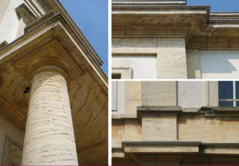
Fig. 4 - Columns, frames and other architectural elements finished with decorative concrete simulating travertine (photo Alvisi 2014).
